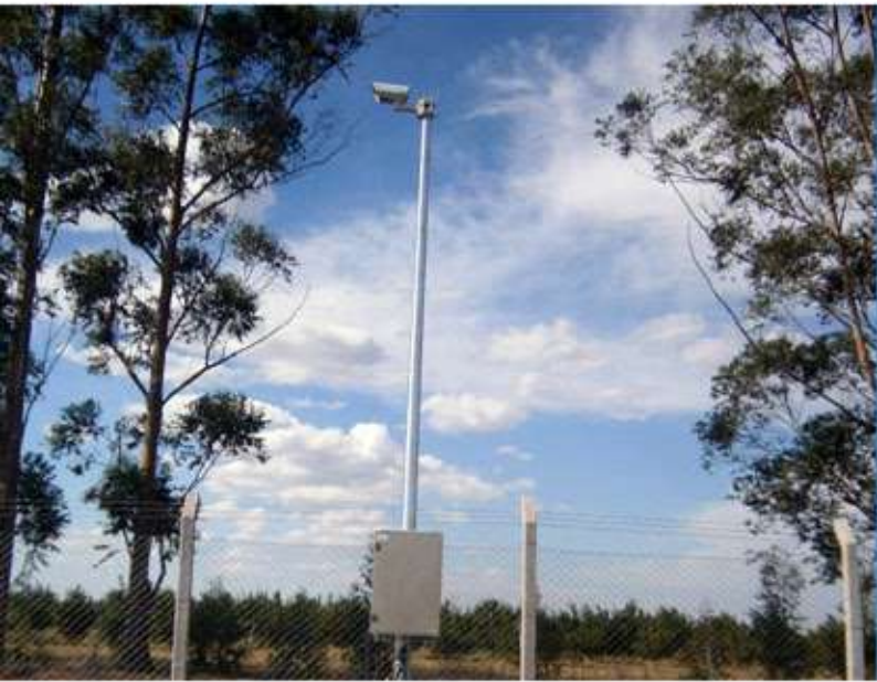
La Jacinta Photovoltaic Plant
