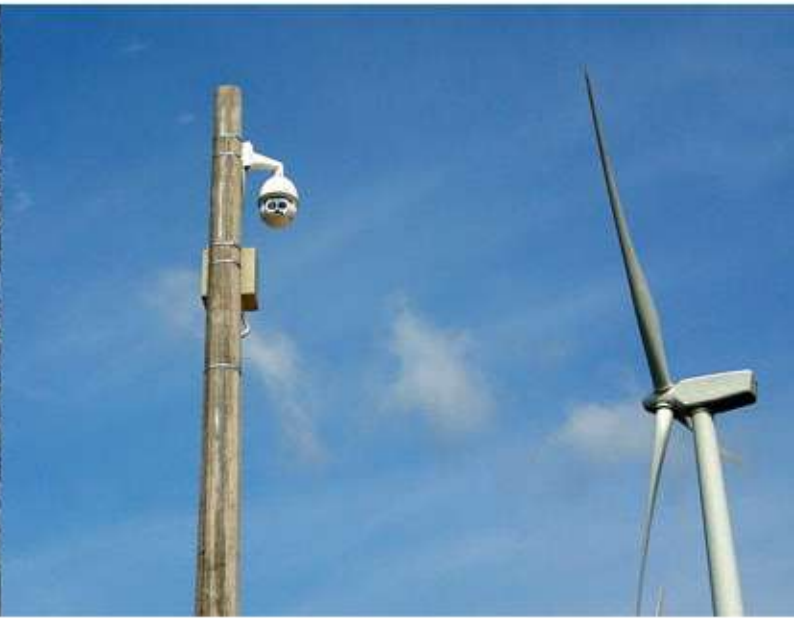
Piedras Largas II Wind Farm
